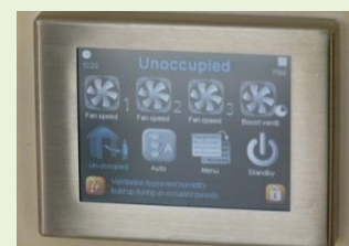
Figure 21: MVHR touchscreen control panel
