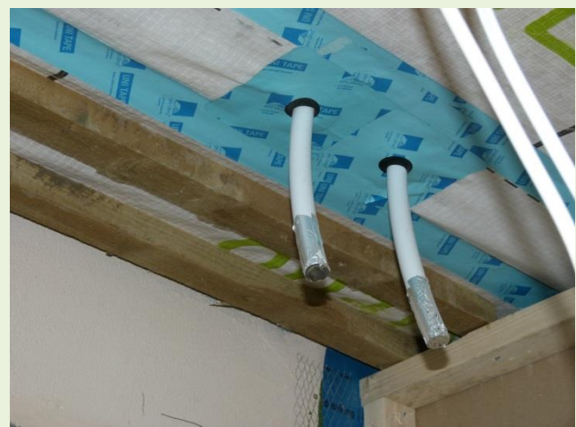
Figure 14: grommets and seals on penetrations
